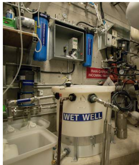
CIRS building rainwater treatment equipment
